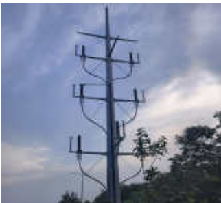
Cable Termination Pole
