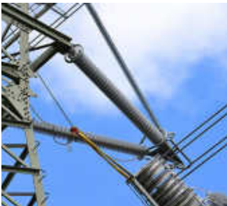
Pole with Insulated Cross-Arm
