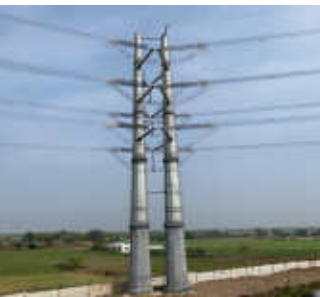
Twin Pole Structure
